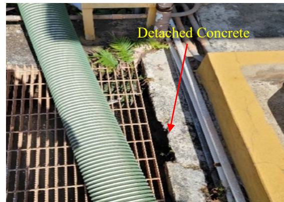
Figure 9 Concrete Detachment on Channel Wall Edge
