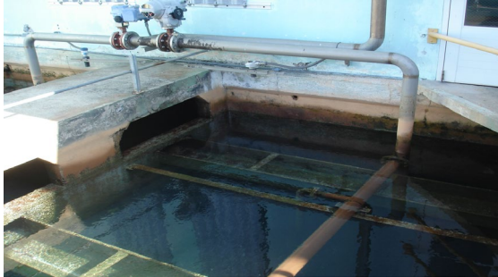
Figure 4 Old Plant Filter #2
