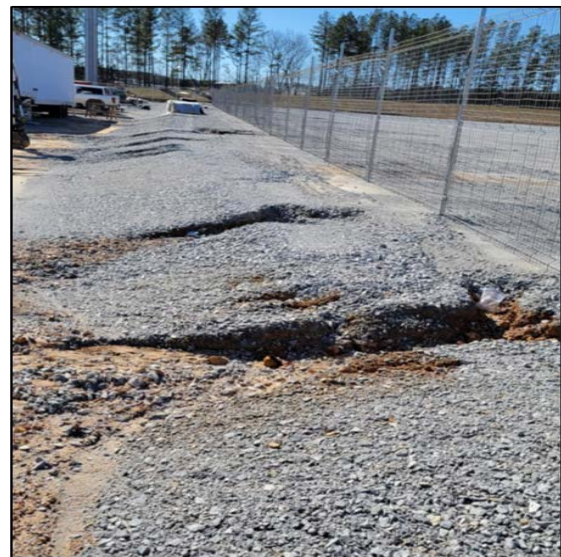
Figure 15 Erosion After Rain Event
